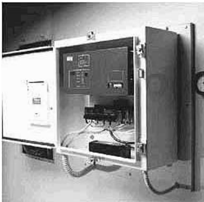
Figure 1. Typical PQNode installation.
