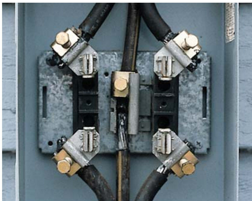
Figure 2 - Photograph of Meter Base
